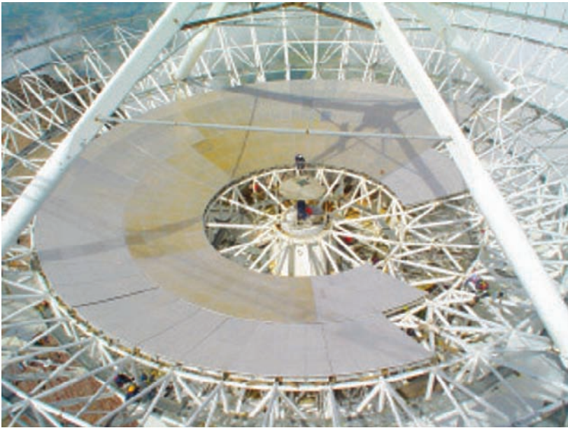
Fig. 7.19. View of the LMT backup structure with the second and third panel ring being installed (Sep. 2006). The approximately 5 \times 2 \text{ m}^2 panels each carry 8 surface plates. Note the yellow dust settled onto the surface at the 4600 m high site. (E. Mendez, INAOE)
