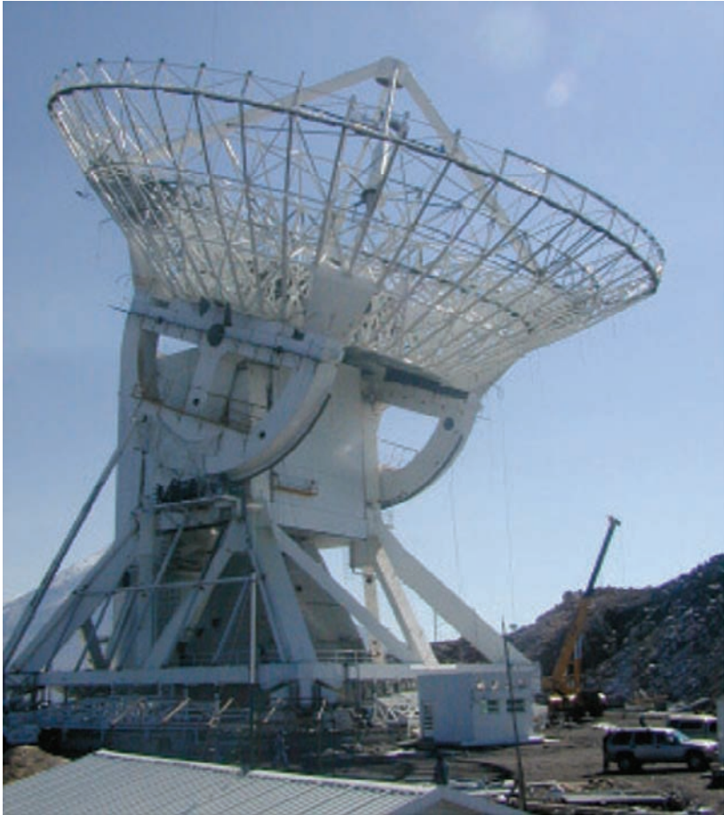
Fig. 7.20. The 50-m diameter LMT under construction at an altitude of 4600 m on Cerro la Negra, central Mexico in summer 2006. (E. Mendez, INAOE)
